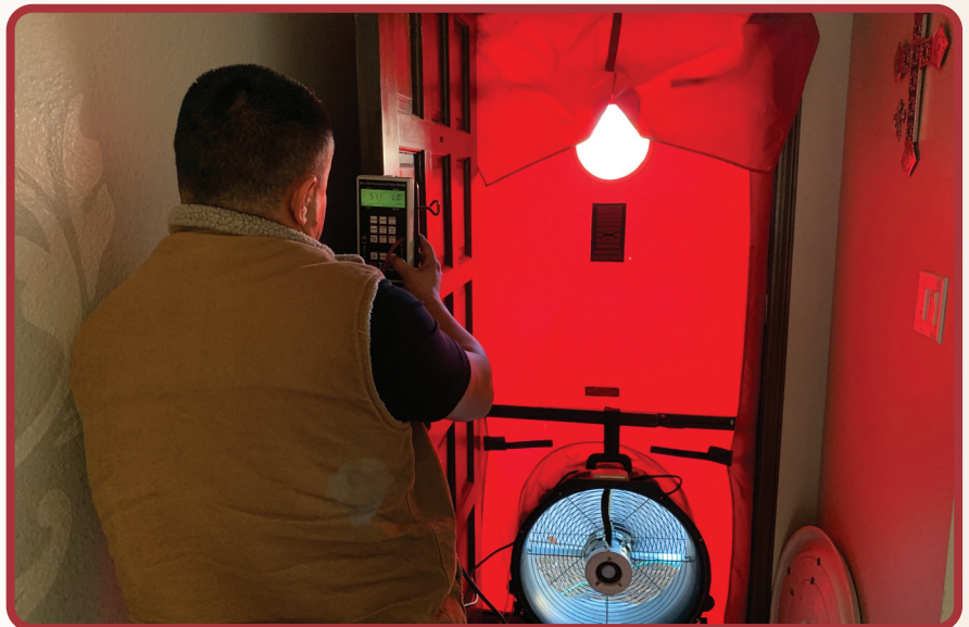
A contractor measures air leaks in a home using a blower door test. This diagnostic tool measures how much air is leaking in or out of a home, and reveals areas where air sealing will help make a home more energy efficient.
